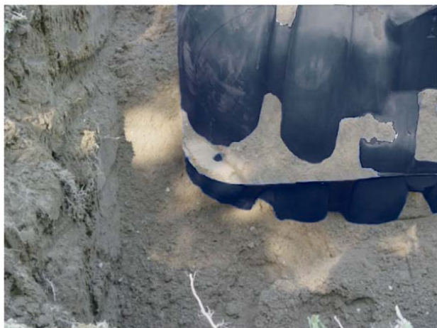
Photo 4.1.7-Proper support for vessel
